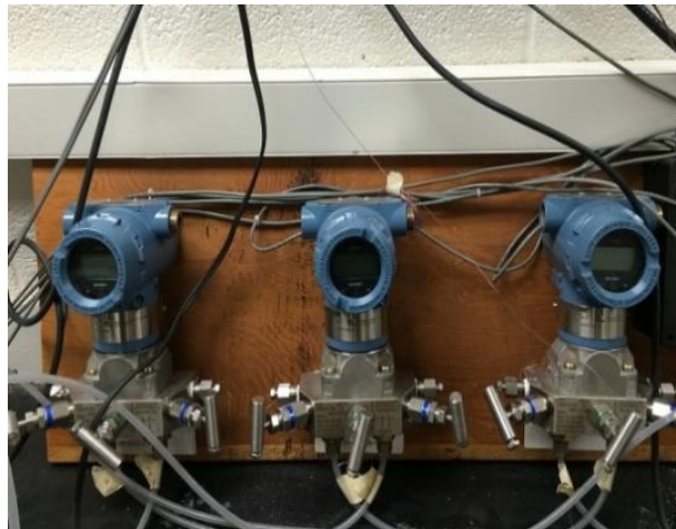
Figure 3.5 Three Rosemount pressure transmitters (model 3051) connected in parallel.
