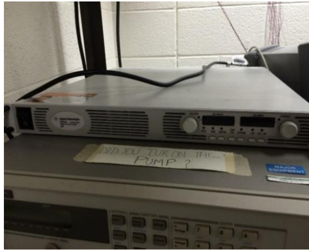
Figure 3.8 N5761A Agilent DC power supply unit.
